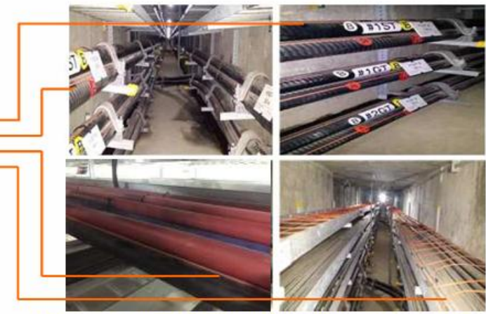
< Application example of optical fiber temperature measurement system >
